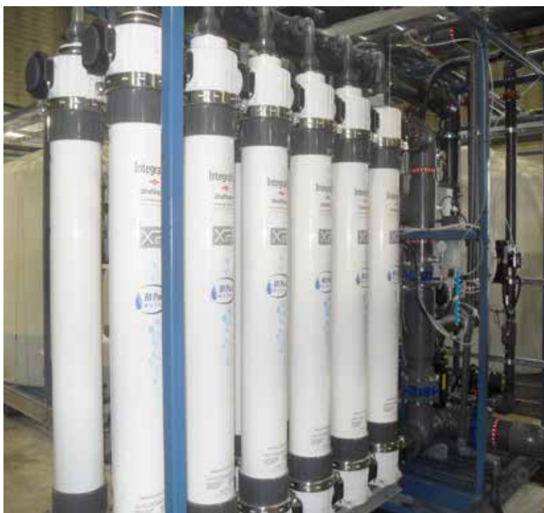
The primary and secondary filtration featuring Dow ultrafiltration membranes
