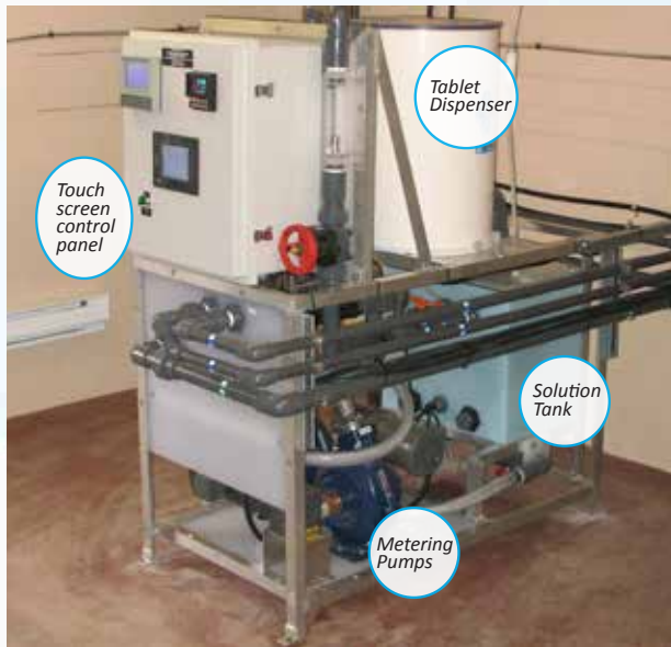
Nine BI Pure Water calcium hypochlorite tablet systems were installed throughout Whistler for the 2009 Winter Games; seven are still being used.
