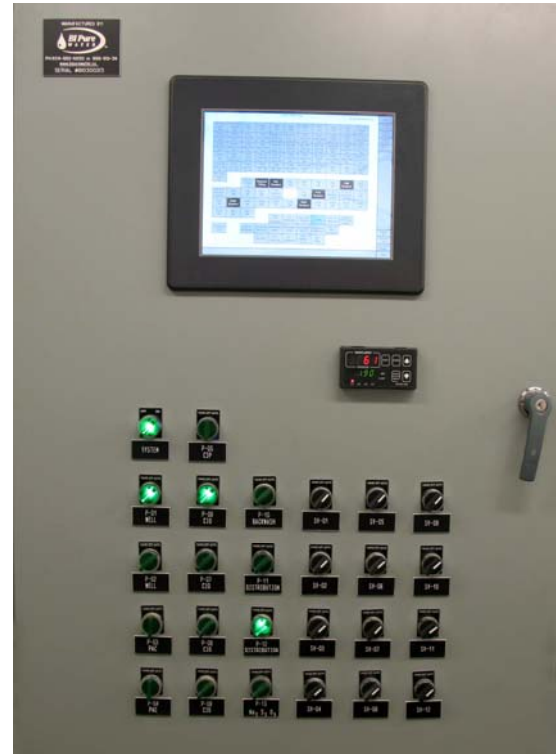
The control panel provides redundant controls
