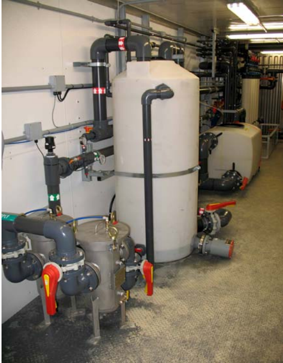
Inlet screen filtration and CIP tank
