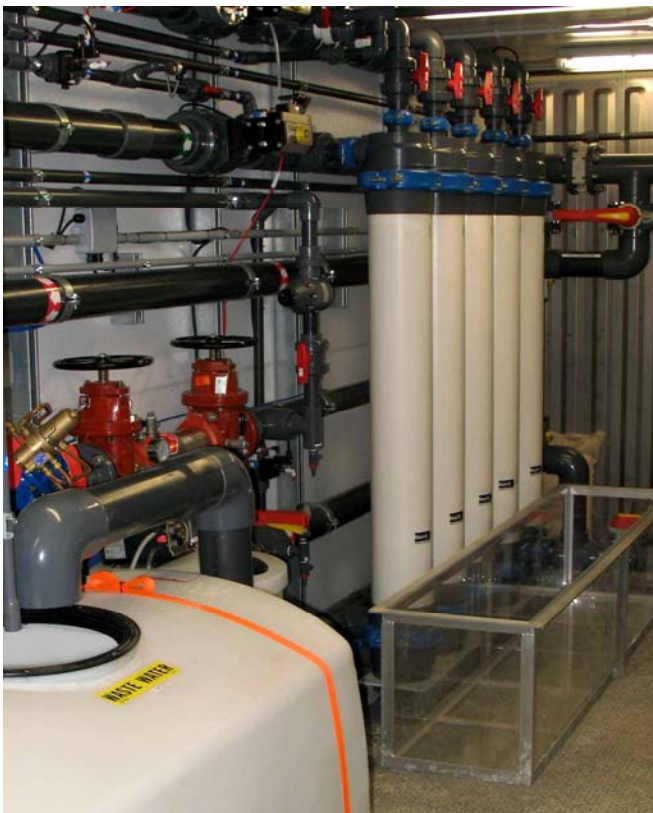
Five UF housings are mounted on each side.
