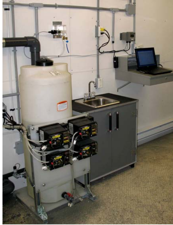
Metering pumps for chlorine injection
