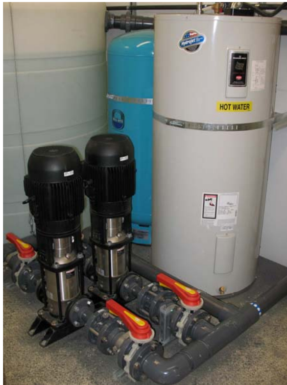
Distribution pumps move water from storage
