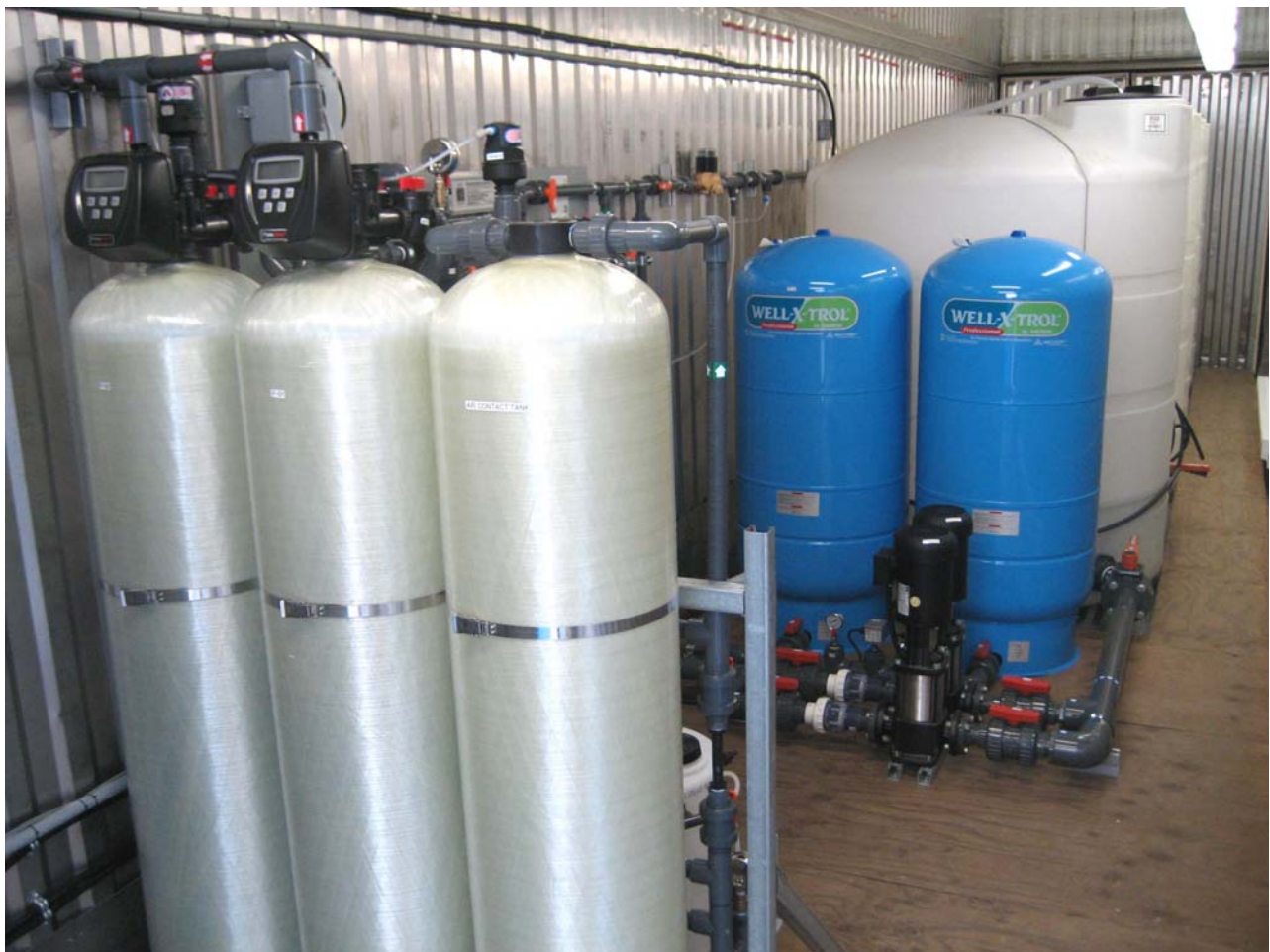
Picture of the interior of a typical containerized package plant provided to NovaGold/Teck.
