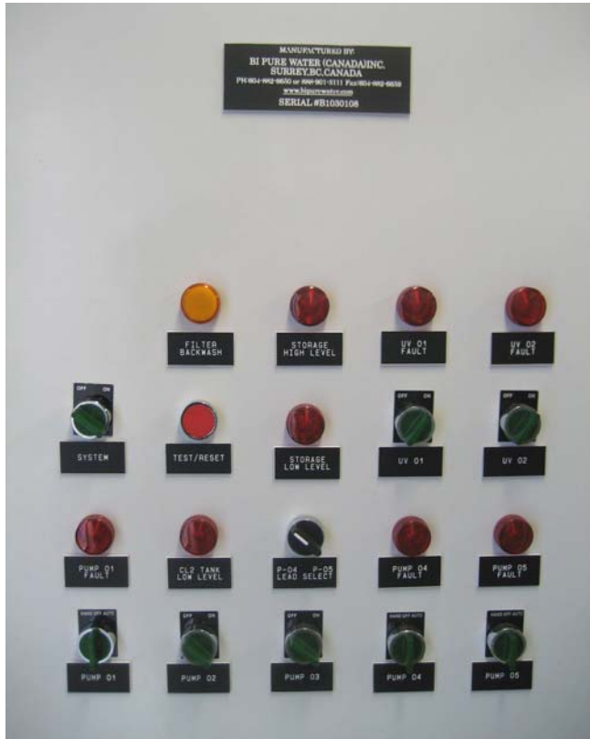
Typical control panel for the water treatment plants supplied to NovaGold/Tech Cominco.
