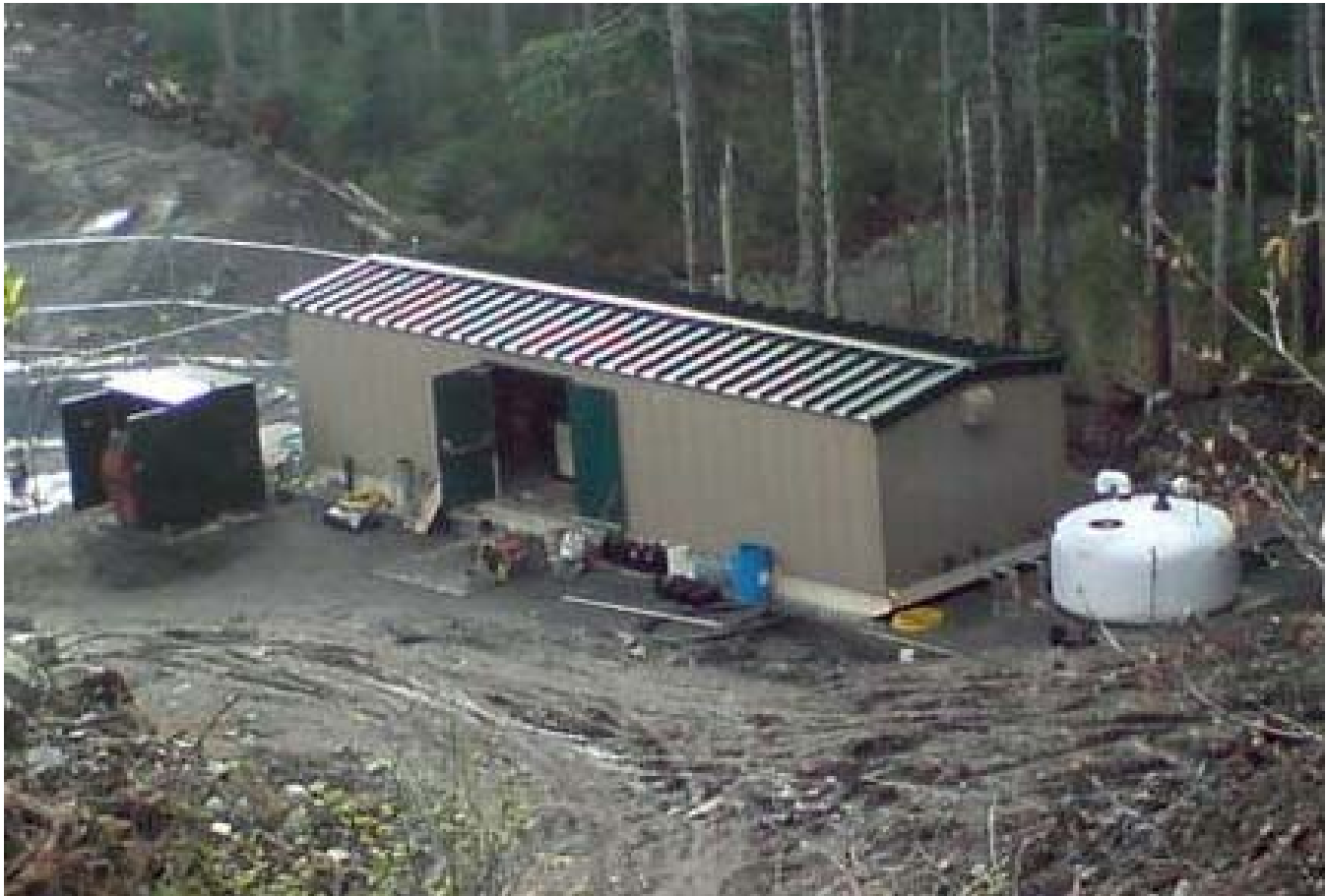
Figure 1 – The water treatment plant was skidded to its location above the community
