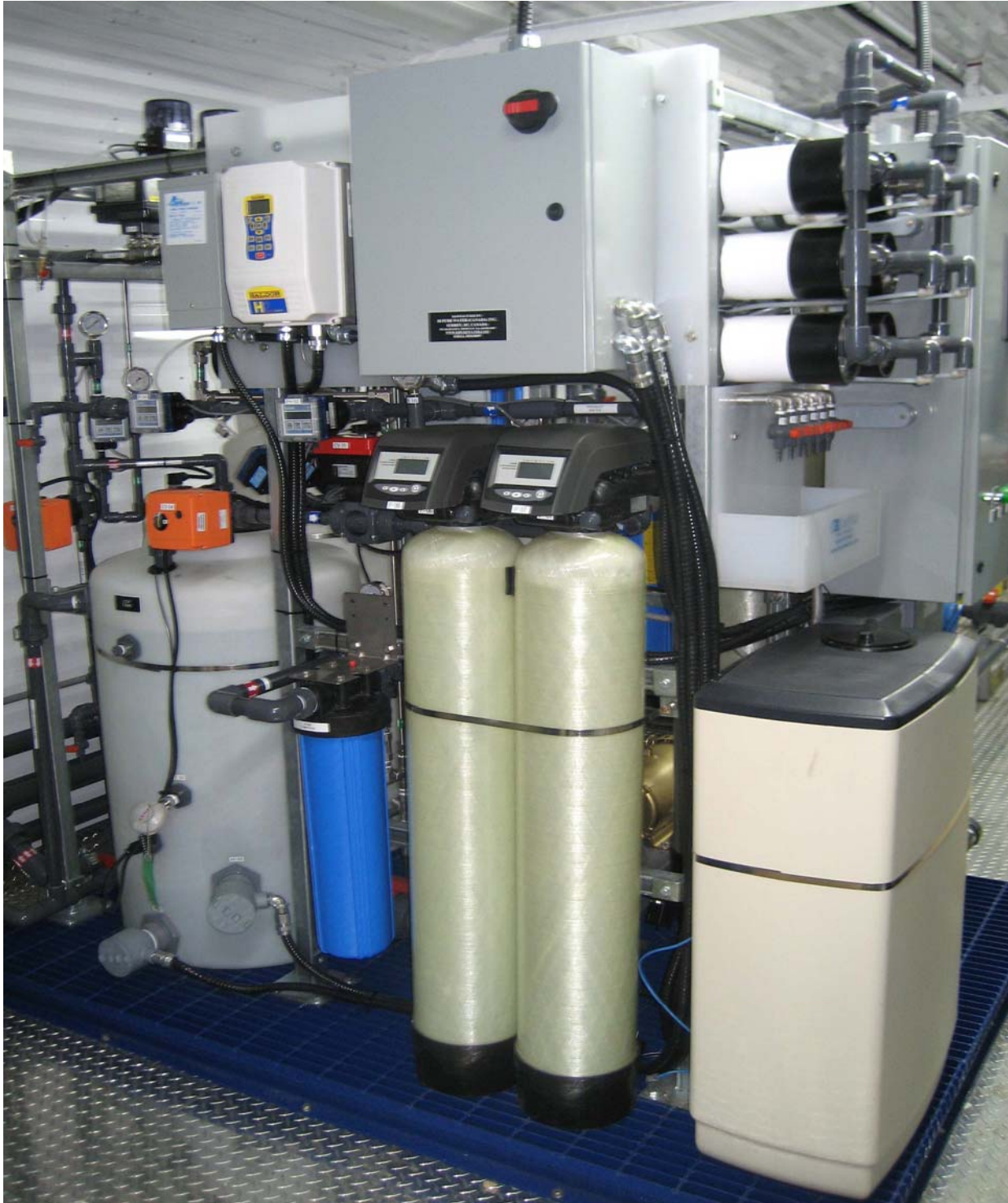
Figure 2: The BI Pure Water Reverse Osmosis Water Treatment Plant under study
