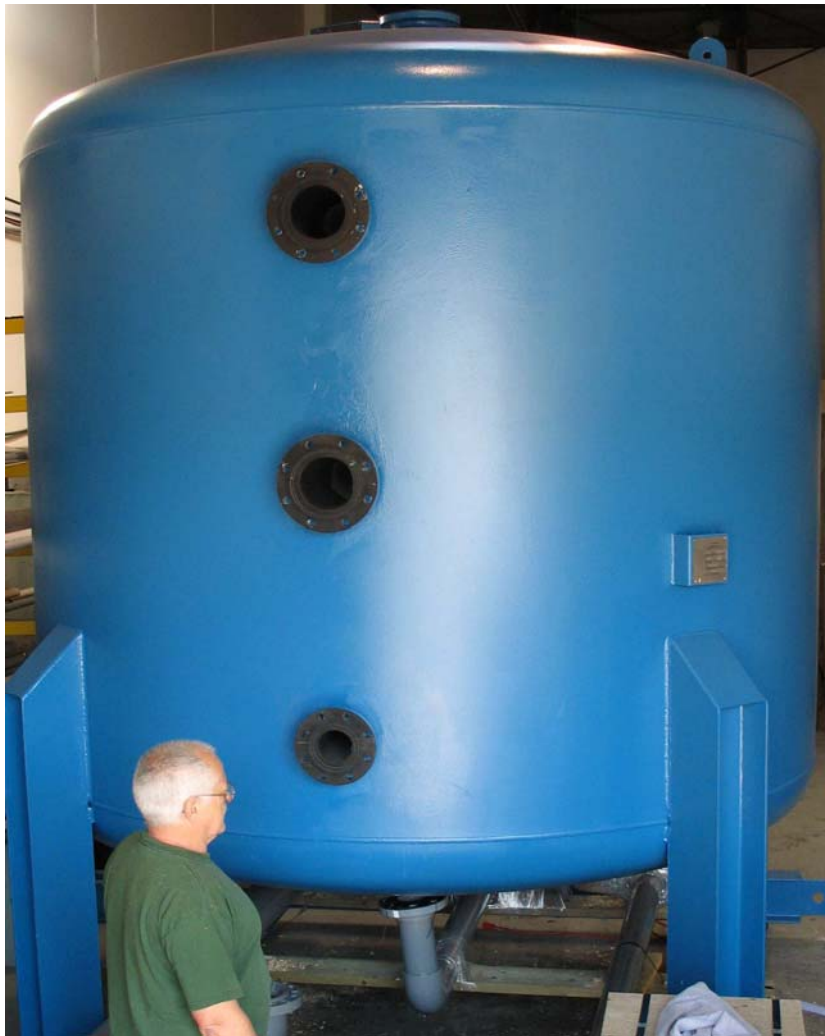
Figure 2 - Big Boy 108 inch diameter steel media vessels.
